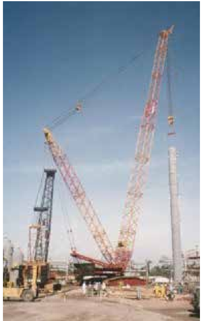
Lifting a 95 tons pressure vessel with the Demag CC-4800 of Van Seumeren at the GPP-4 plant, Kerteh, Malaysia, 1994
