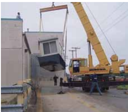
Fig.13 Unstable load, due to using wrong type of lift beam
